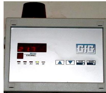
Permanent O 2 measuring devices
